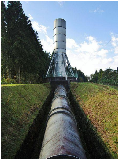
Figure 3: Steel Surge Tank at Isawa II Power Station in Japan
