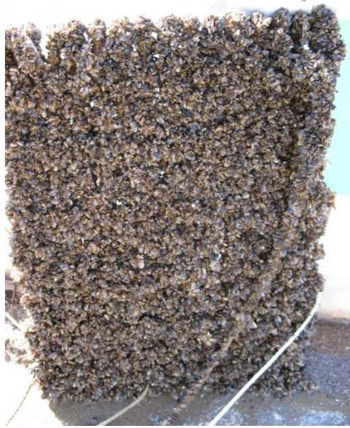
Figure 4: Invasive Zebra Mussels on Steel Surface
