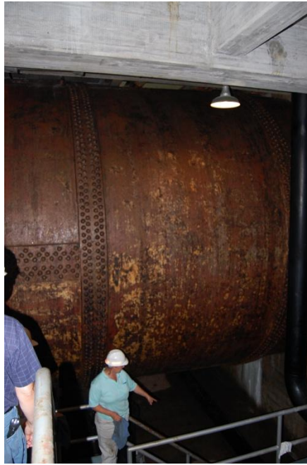
Figure 5: Exposed Portion of Penstock at Center Hill Hydro Plant in DeKalb Co., Tennessee
