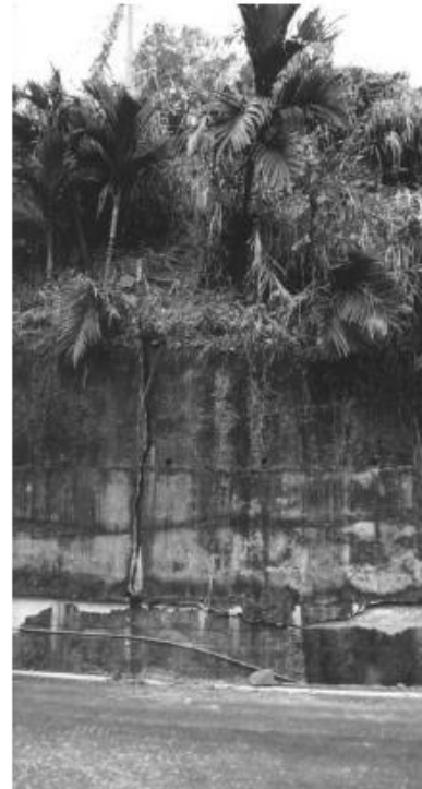
RETAINING WALL FAILURE
