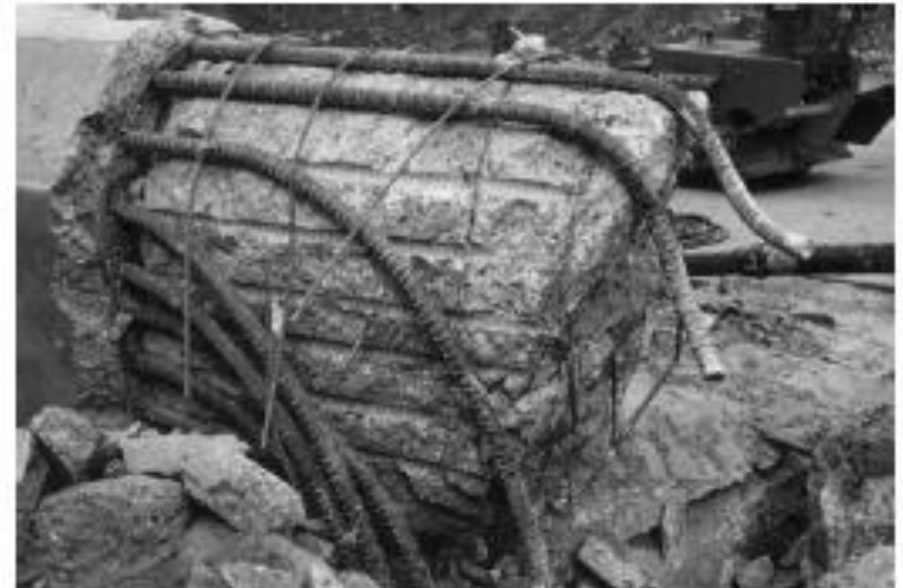
FOUNDATION JOINT FAILURE
