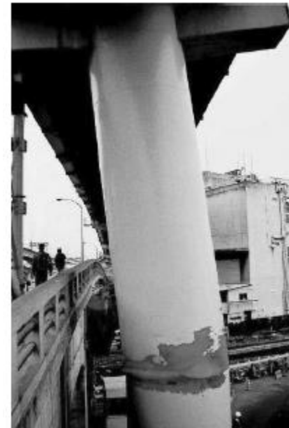
STEEL COLUMN BUCKLING
