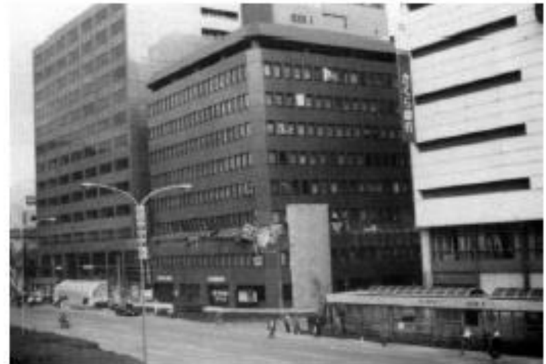
SOFT STORY AT 3 RD FLOOR
