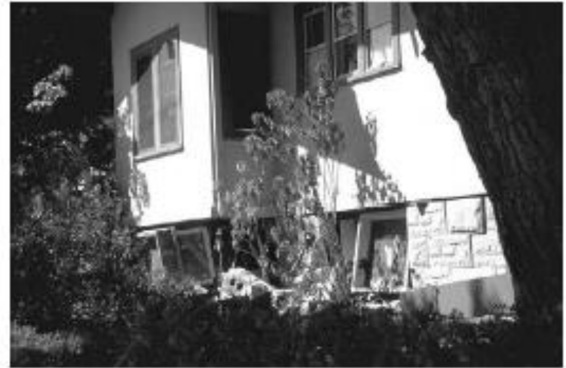
MASONARY BLOCK FAILURE
