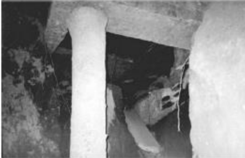
SOIL WASHED OUT DUE TO BROKEN PIPES UNDER GROUND
