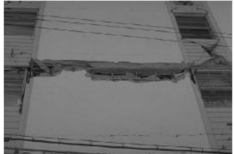
SHEAR WALL FAILURE
