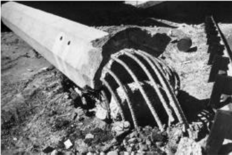
PILE FAILURE AT FOUNDATION JOINT
