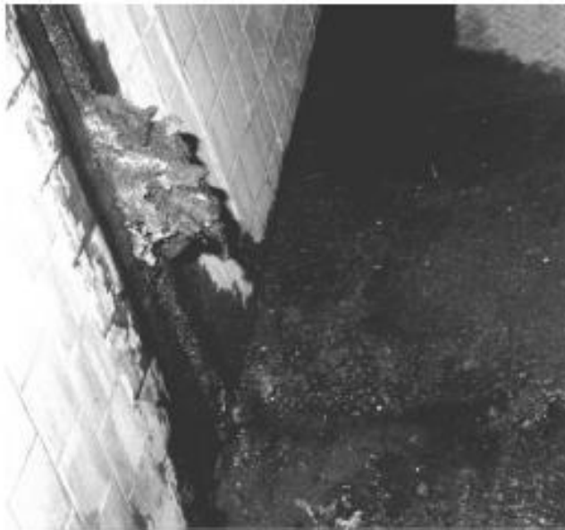
LIQUEFACTION OF SOIL FAILURE
