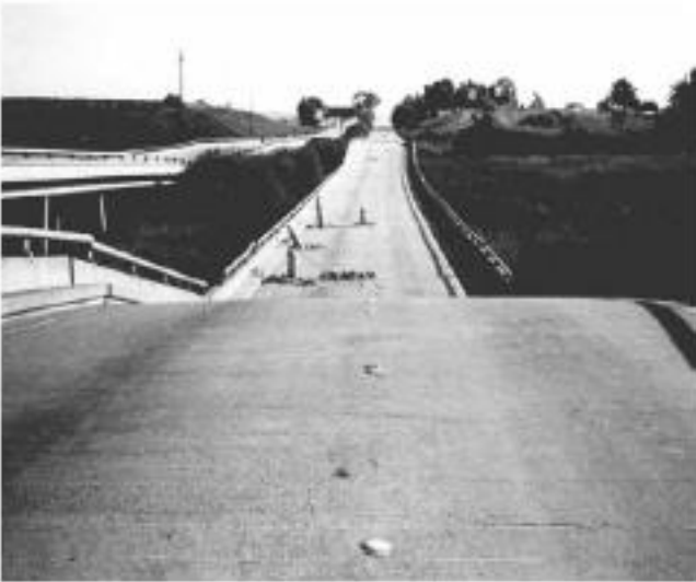
PILES POPPING DECK SLAB
