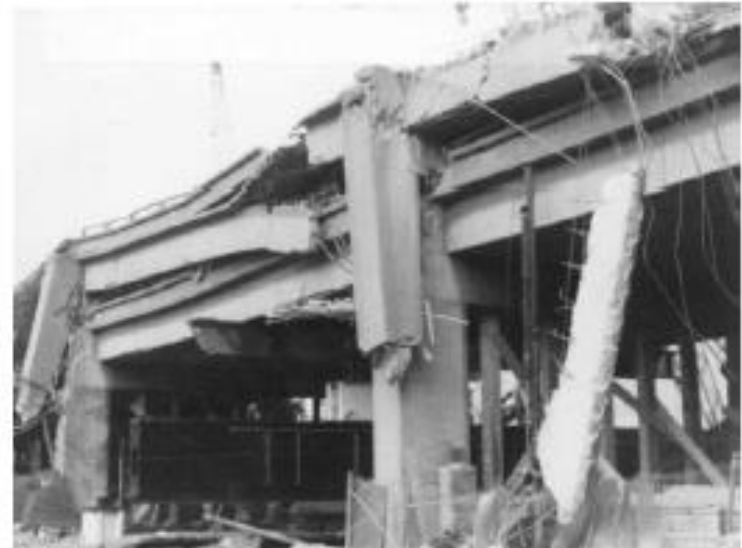
FOUNDATION JOINT FAILURE
