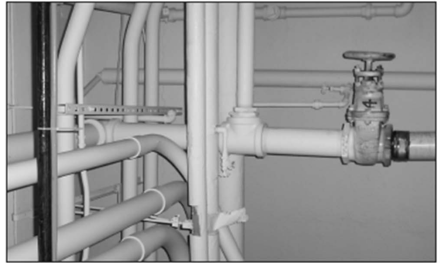
Piping and plumbing systems
