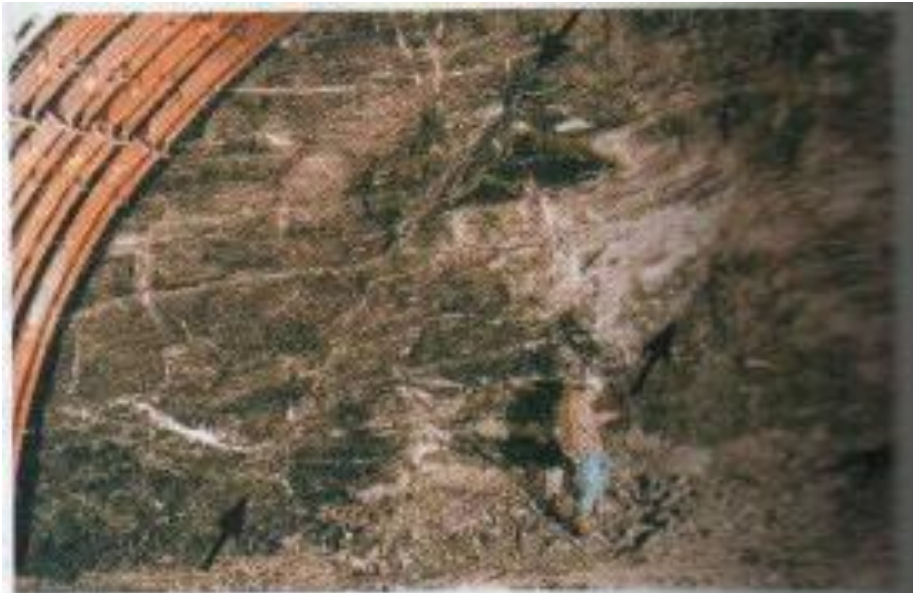
Figure 10.34 Faults intersecting the tunnel excavation front in RMR Class IV shales.
