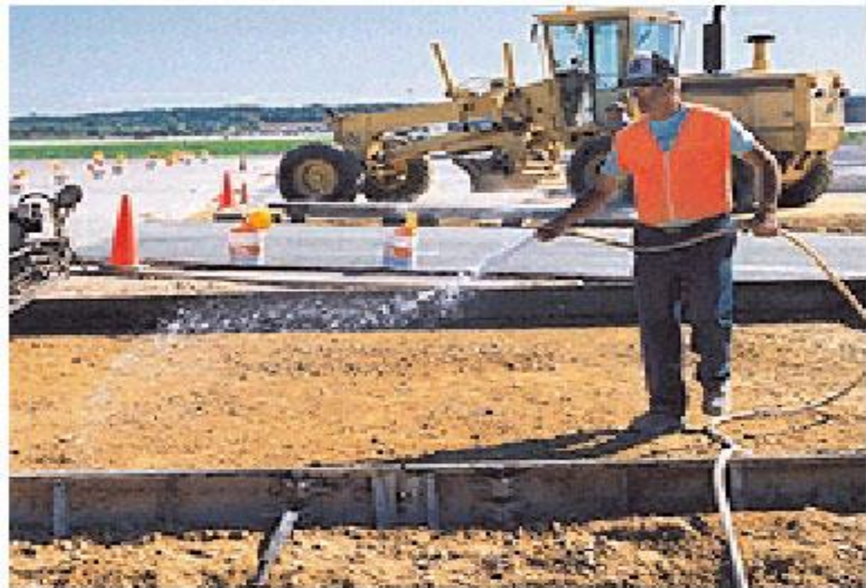
Fig. 13-9. Dampening the subgrade, yet keeping it free of standing water will lessen drying of the concrete and reduce problems from hot weather conditions. (69955)
