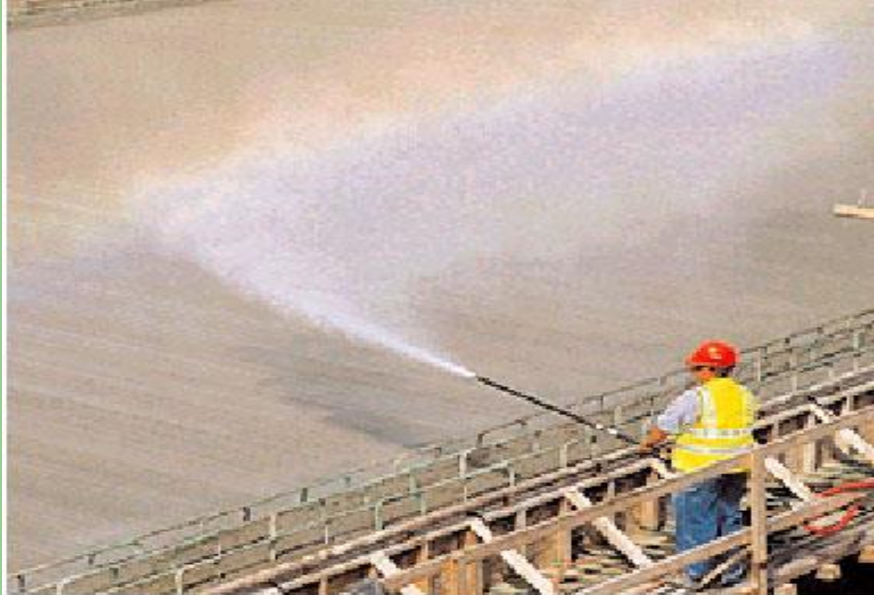
Fig. 13-11. Fogging cools the air and raises the relative humidity above flatwork to lessen rapid evaporation from the concrete surface, thus reducing cracking and improving surface durability. (69956)
