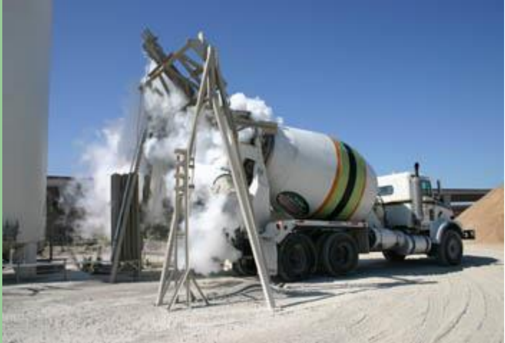
Fig. 13-1. Liquid nitrogen added directly into a truck mixer is an effective method of reducing concrete temperature for delivery to mass concrete placements or during hot-weather concreting. (69954)
