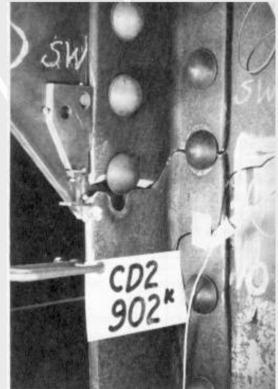
Fracture in Net Area
