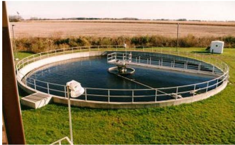
Figure 2-11: Secondary settling tank
