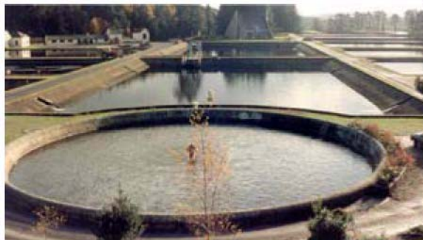
Figure 2-19: Sewage oxidation ponds
