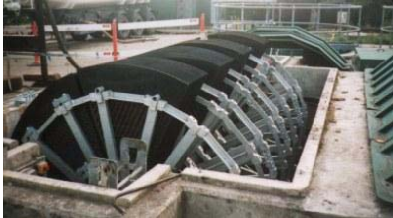
Figure 2-16: Rotating biological contactor
