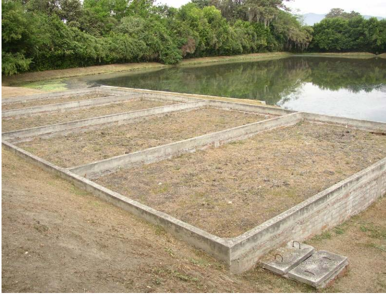
Figure 13. Sludge drying beds at a WSP site in Colombia.
