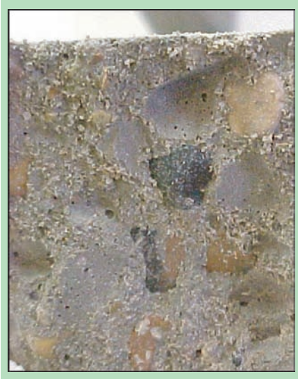
Figure 4.48 Saturated dense concrete.
