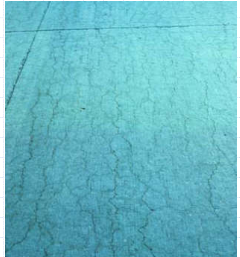
AAR Induced Cracking in Concrete Pavement.
