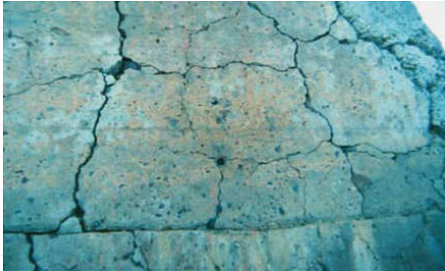
Map cracking pattern Bridge Pier, Medicine Hat, Alberta
