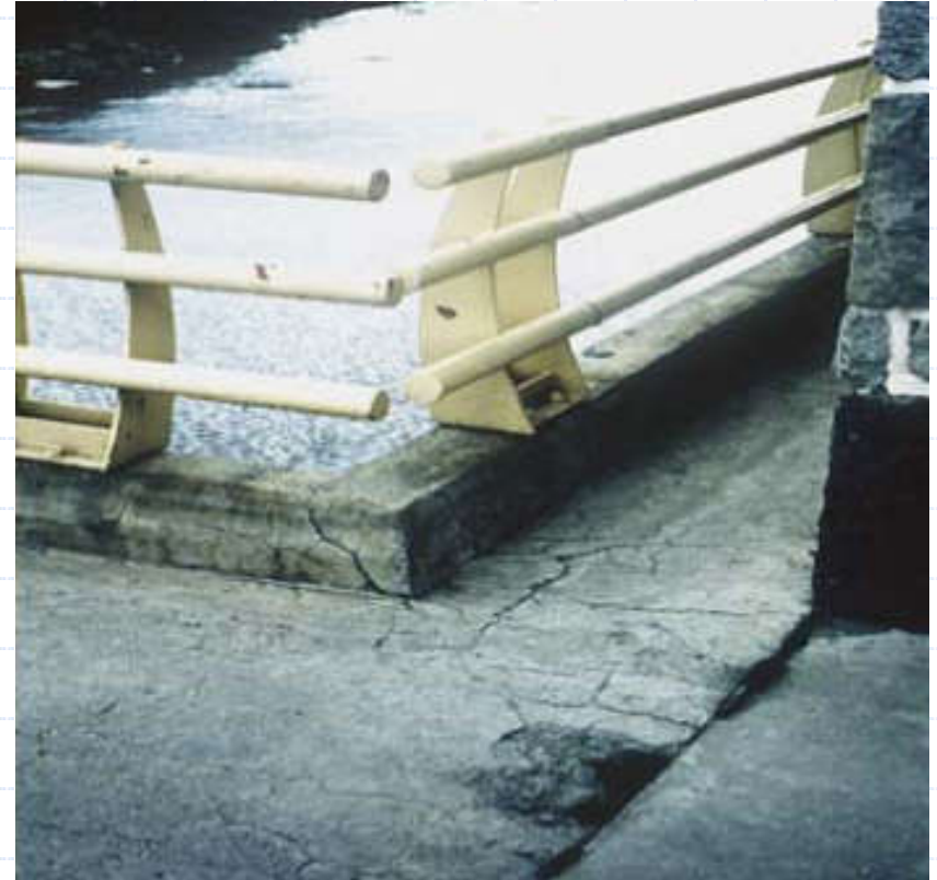
Displacement caused by ASR-induced expansion in bridge structure; spalling and extrusion of jointing material
