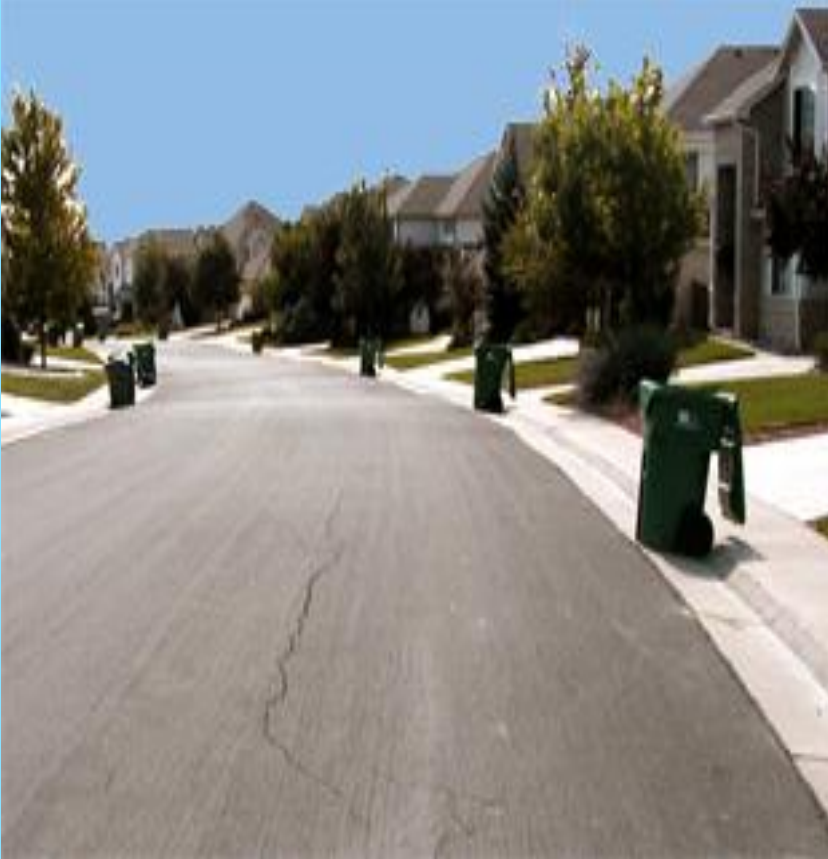
Cracks in Pavement
