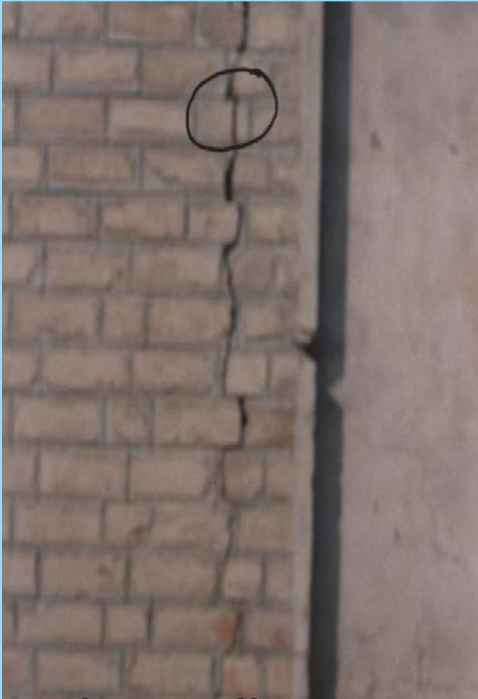
Crack in Wall
