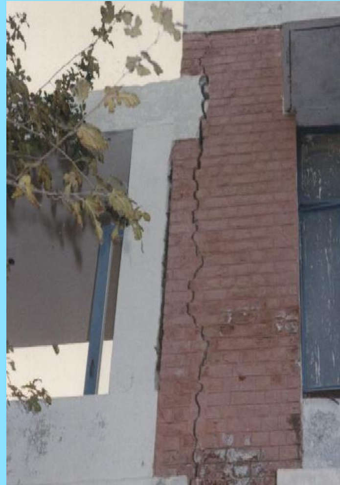
Cracks in Exterior Wall
