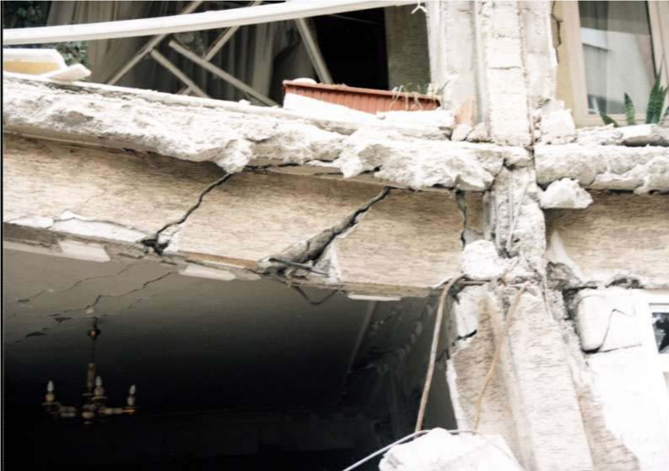
Pure Shear/Web Shear Cracks
